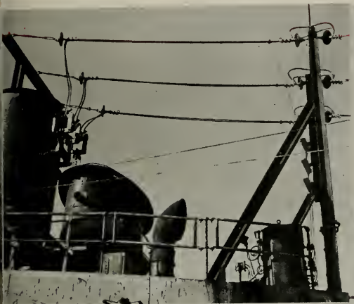
Transmission lines on the SS Donbass at Eureka rigged to carry off power to the main system via transformers installed on the dock.
